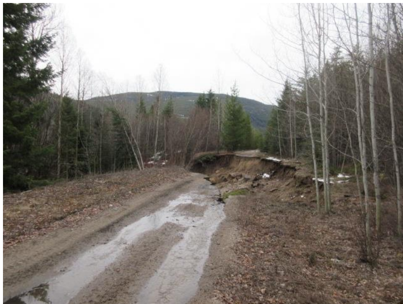
Photo: Rob Miller, Hayes Creek Fire Department
